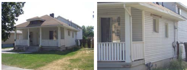
Vinyl is not appropriate as a primary material for bungalows; however, it may be fine to use for soffits and less-visible portions of the elevation.
