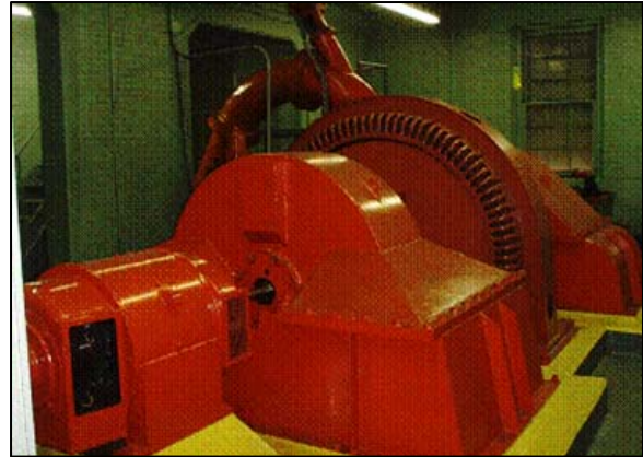
Figure 7-10 The Hobble Creek Hydro is located just west of the Hobble Creek Golf Course #6 Tee box on Hobble Creek.
